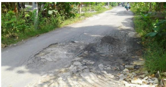
Figure 5. The road damage around the connecting roads of Semin District, Gunungkidul Regency, and Sukoharjo Regency.
